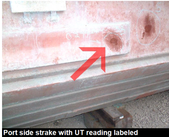
Port side strake with UT reading labeled
